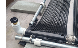
COLLARS ON EVERY RAIL CONNECTION TO BALLAST MADE OF 1.5" PVC SCH 40 PIPE
